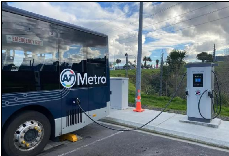
Figure 21: Example of Typical Bus Depot Charging
