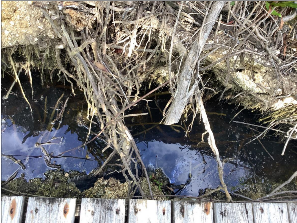
Photo 24: Standing water adjacent to southern boardwalk. (July 2023)
