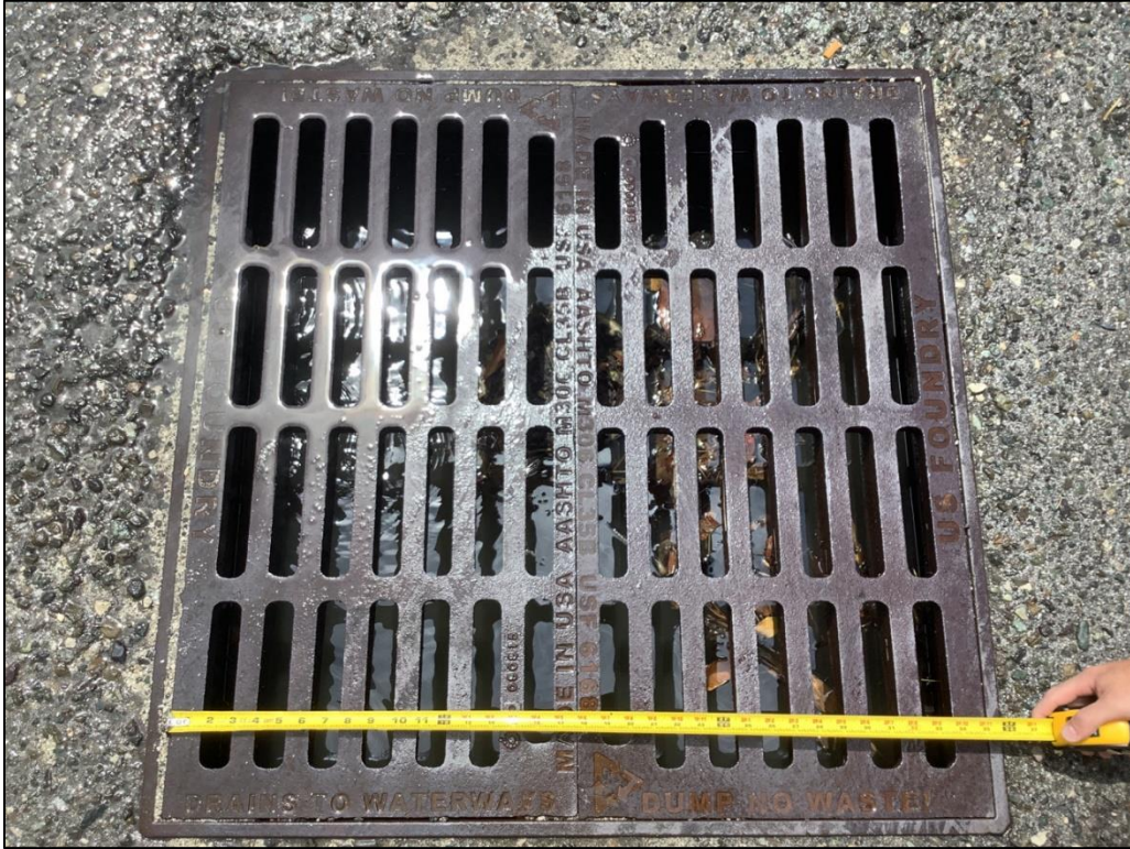
Photo 7: Made in USA inlet (July 2023)
