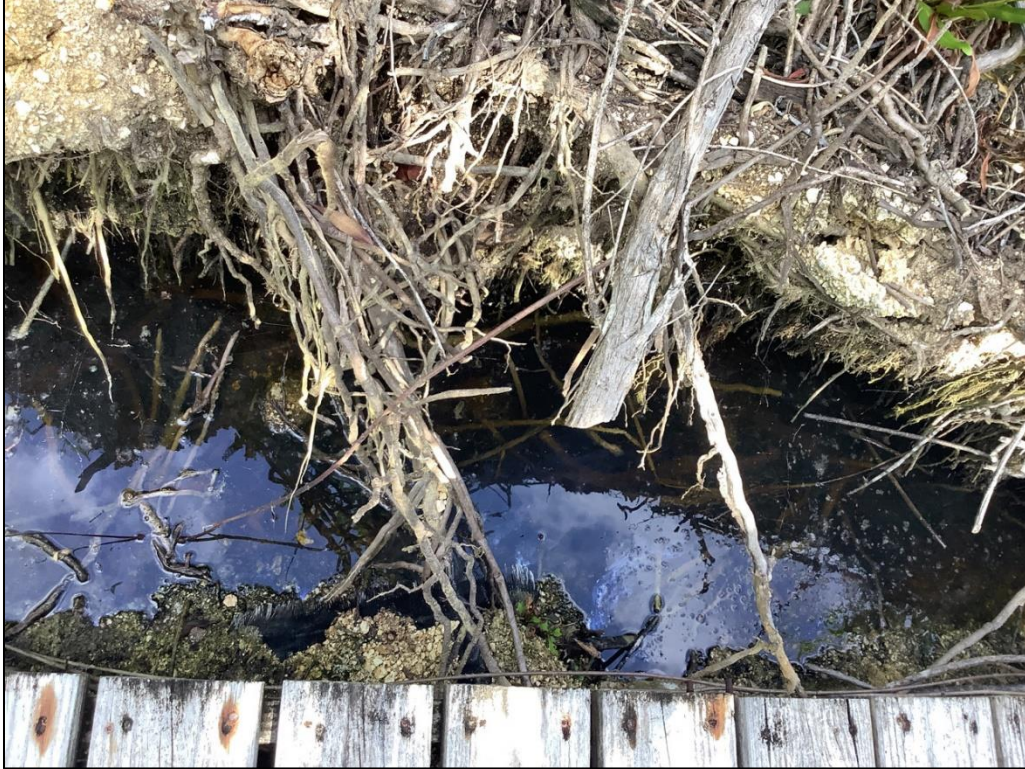
Photo 32: Standing water adjacent to southern boardwalk. (July 2023)
