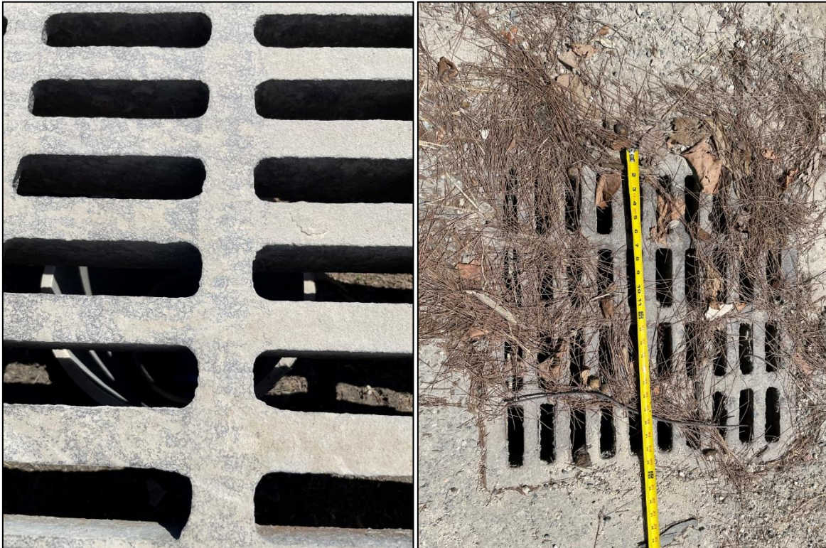
Photo 9: Inlet clogged with sediment (top) and debris (bottom) (July 2023)
